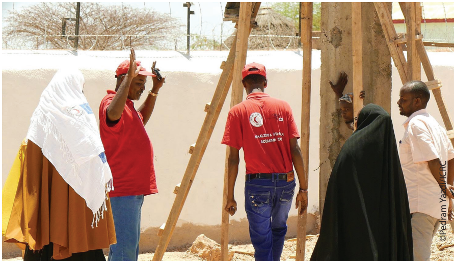
Abdulkadir Hussein (hands raised), branch secretary for SRCS Huddur tours the premises with volunteers during construction of the new SRCS building.
